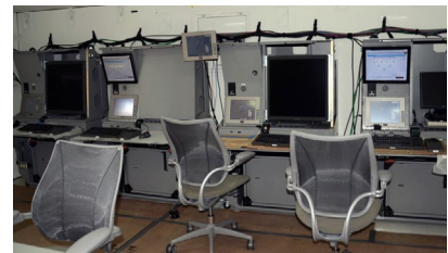
Operations Shelter interior
